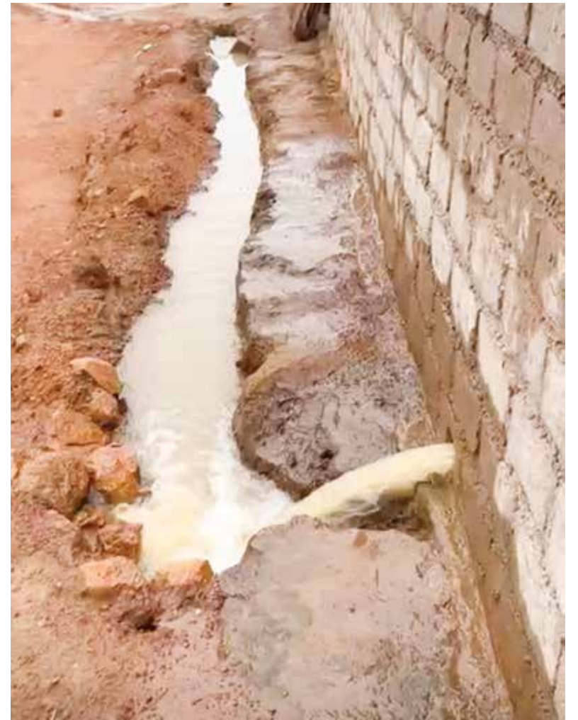
Tafelkop Mall management has denied claims of sewer spillage into nearby residences, citing that the problem as a mere storm water overflow.
