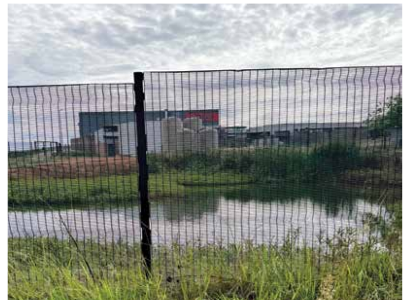
The Tafelkop Mall management is refuting claims that the mall's sewer system is overflowing to the nearby residential area, claiming that the issue is actually caused by storm water overflow.
